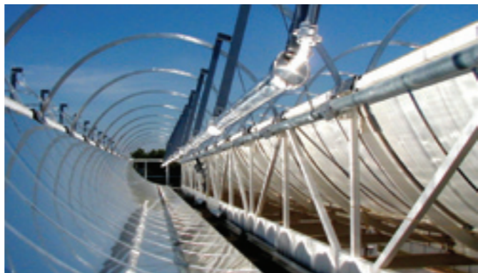
Detail of the Liddell solar thermal power plant .
